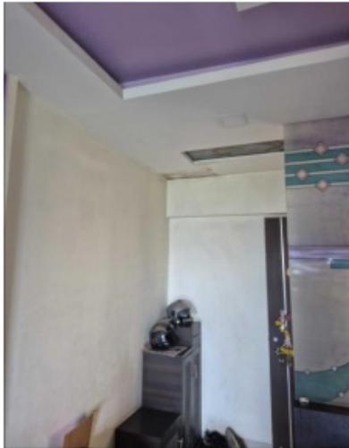
Live moisture on ceiling
