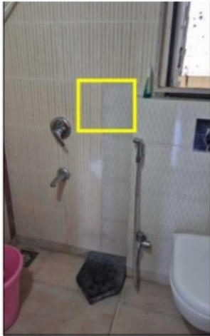
Leakage from pipe line
