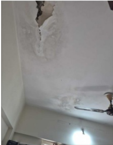
Water dripping from ceiling
