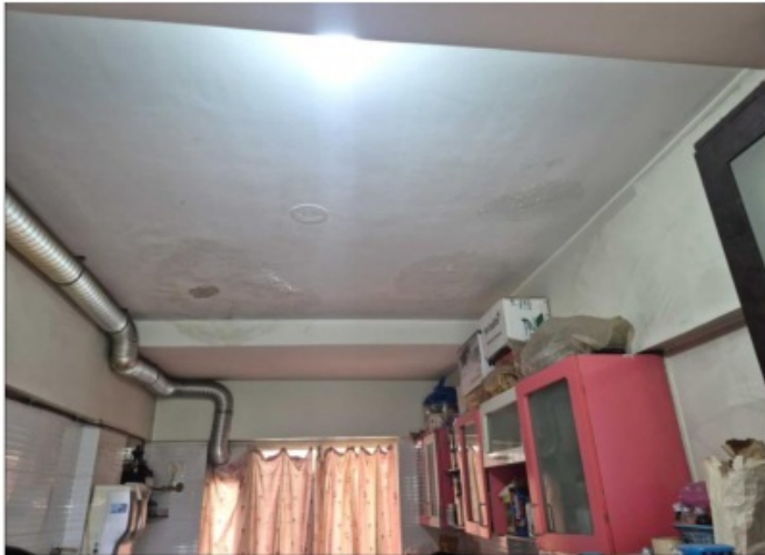
Water dripping from ceiling
