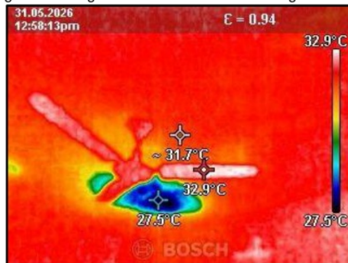
Thermal image of water dripping from ceiling
